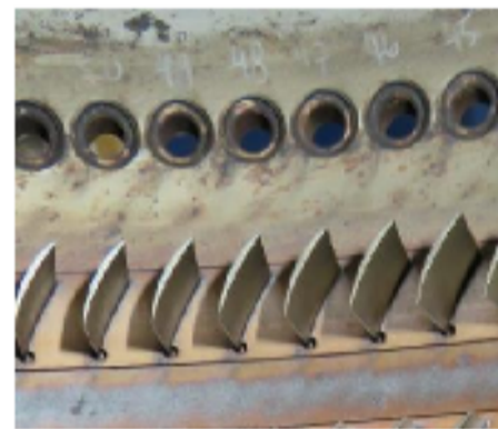
DISASSEMBLY CONDITIONS SHOWING CORROSION/PITTING OXIDATION FINDINGS (STAGE 5 AND STAGE 6)
