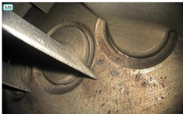
STAGE 5 CORROSION/PITTING INDICATION EXAMPLE
