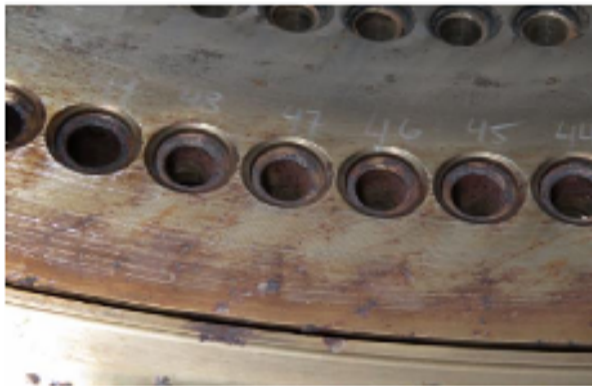
DISASSEMBLY CONDITIONS SHOWING CORROSION/PITTING OXIDATION FINDINGS (STAGE 5 AND STAGE 6)
