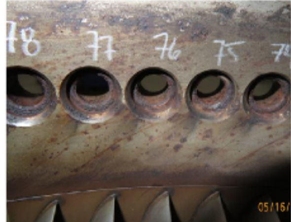
DISASSEMBLY CONDITION CORROSION PITS IN THE SURFACE OF INNER COMPRESSOR + EXAMPLE OF CORROSION IN VANE BORES
