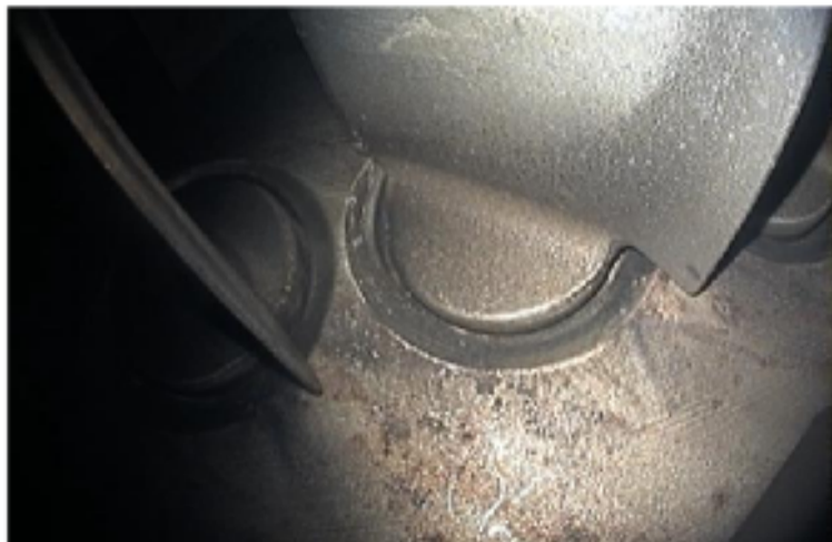
STAGE 5 CORROSION/PITTING INDICATION EXAMPLE
