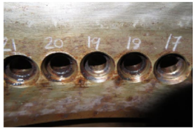
DISASSEMBLY CONDITION CORROSION PITS IN THE SURFACE OF INNER COMPRESSOR + EXAMPLE OF CORROSION IN VANE BORES
